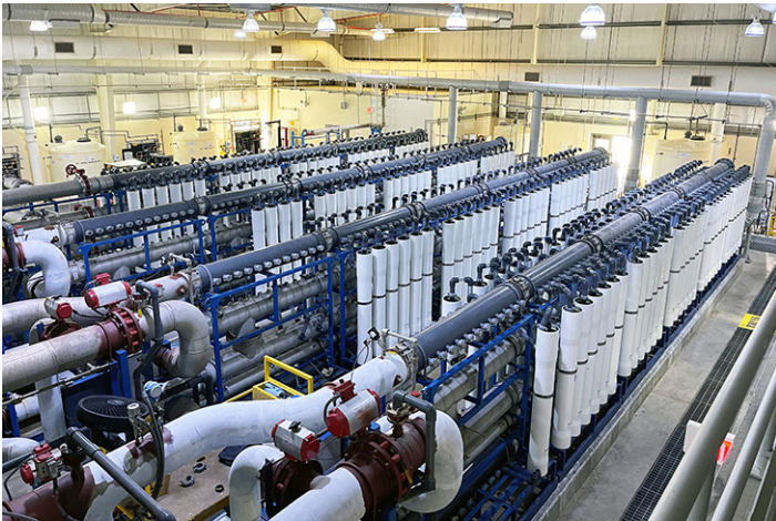
KCUD WTP following Ultressa ceramic UF retrofit – Note capped fittings on filtrate header, which previously accommodated original modules
